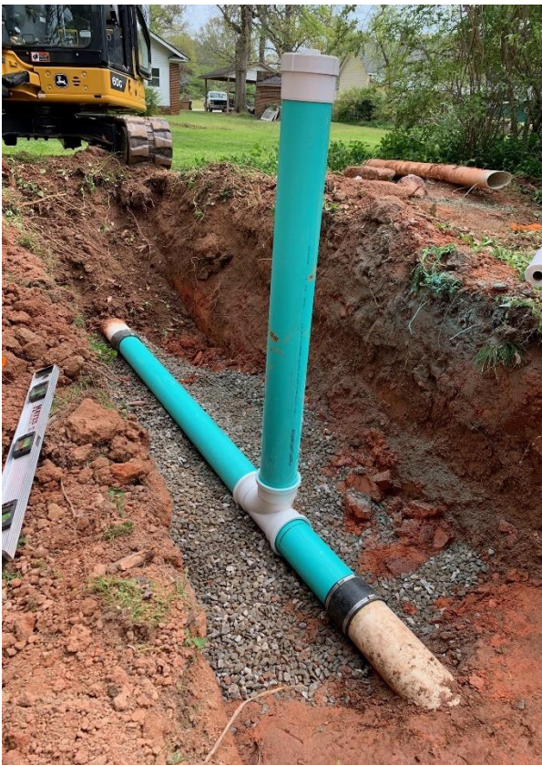
Left – Sewer line repair in an alley running parallel to Railroad Street. Due to tree roots clogging the line and deforming the pipes, this repair was needed to resolve the issue of blockage. Additionally, by adding a “T” and cleanout allows for more efficient maintenance in the future.
