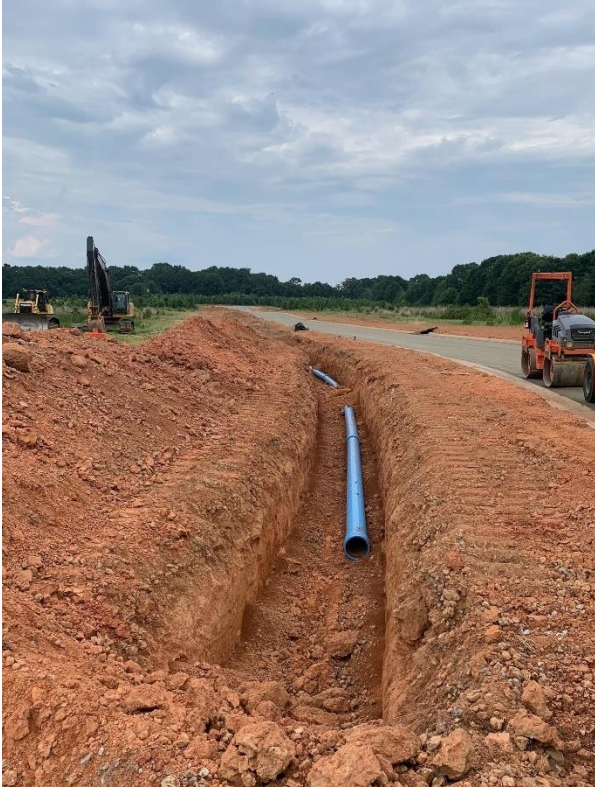
Left - Water line inspection in Springside Meadows Phase III. Inspections such as this are important because it ensures contractors are installing the correct materials, at the correct depth and in the accurate location in the utility corridor.
