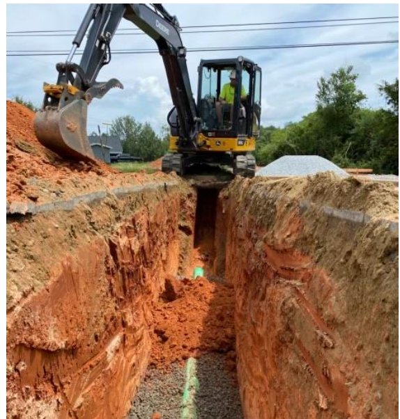
Above – A picture of the recently purchased John Deere Mini Excavator. This piece of equipment is utilized frequently for utility repairs and maintenance as well as a variety of other public works projects.
